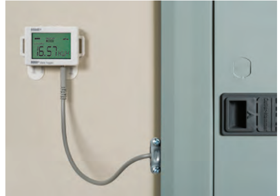
HOB0 UX90-001 State data logger monitoring plug load at the panel
